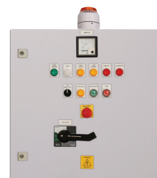
30kW Pump Control Panel
